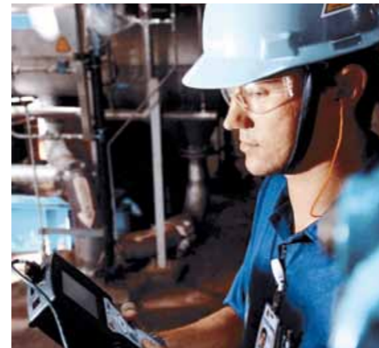
▲ Daniel Scigo, Analytical Supervisor with Sindus Andritz, checks the calibration of digital instrumentation in the new CTMP plant. Sindus Andritz has 40 professionals at work in the Monte Alegre mill complex.
