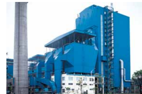
▲ Huaihua's recovery boiler has a capacity of 2200 tds/d. The ANDRITZ recovery unit ensures compliance with international standards for emissions.
