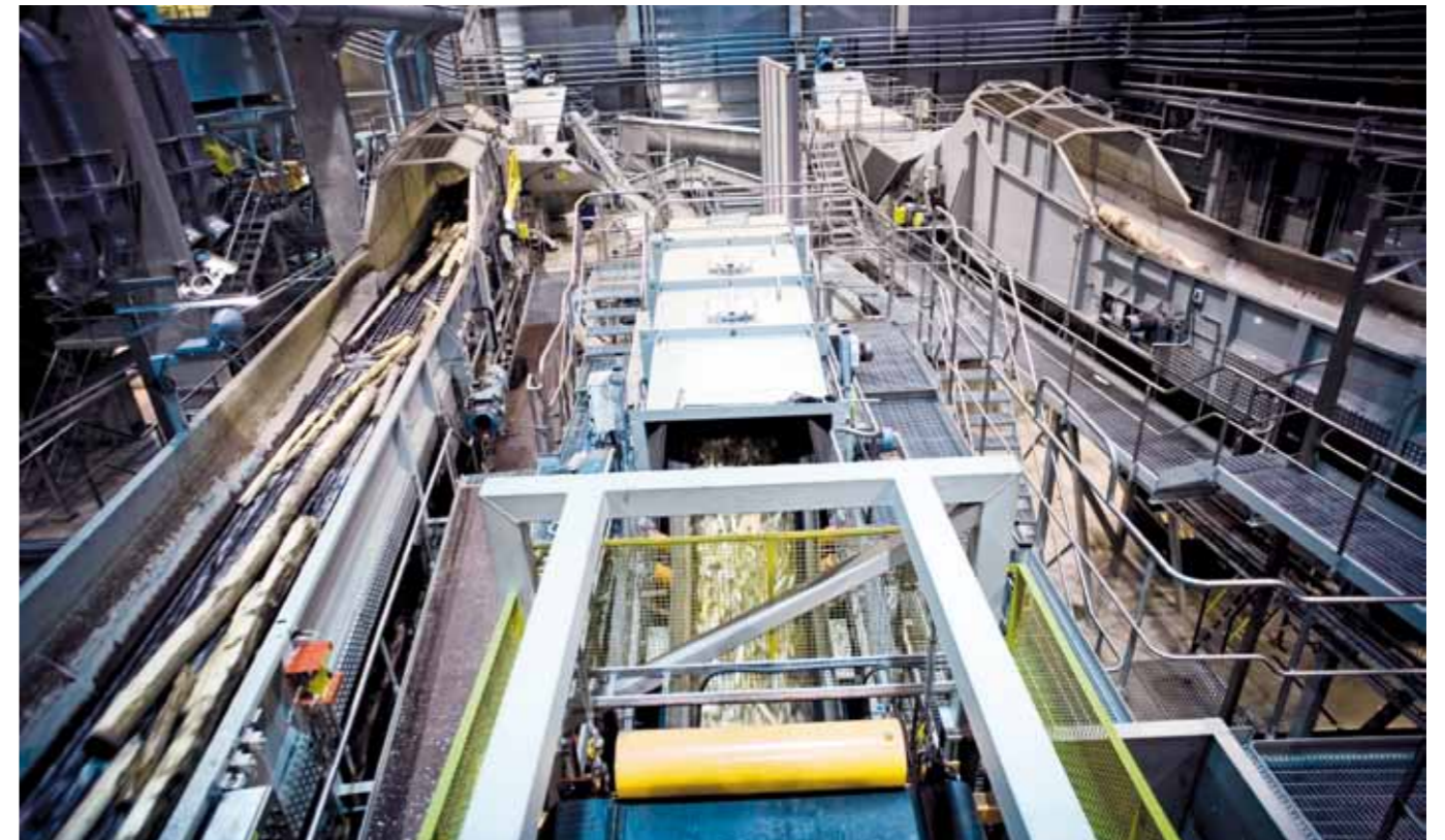
▲ The ANDRITZ woodyard at Varkaus consists of a two-line debarking, chipping, and screening operation. Softwood capacity is 350 m 3 sob/h, while hardwood capacity is 250 m 3 sob/h.
