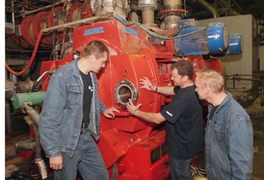
▲ As part of the rebuild of TMP 1, Andritz upgraded the Twin refiners to have Trammable And Guideless (TAG) capability. This allows the mill to adjust the plate gap to ensure that it is parallel over the entire service life of the refiner. Process Engineer Igor Viktorovich Berdjugin (left), Rudolf Hafner of Andritz (center), and Aleksey Iwanchin, Deputy Head of TMP Production at Solikamsk, inspect the refiner rebuild.
