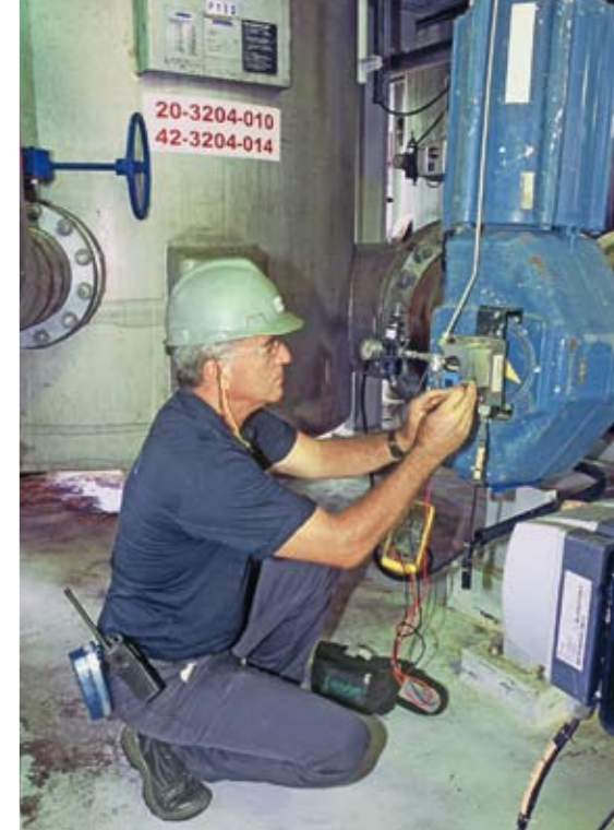
▲ Based upon the input from the OPP system, it was determined that the bad control loop was due to a faulty valve positioner. Here Nelson Vaverro of Sindus Andritz performs a test on the instrument to confirm the problem.
