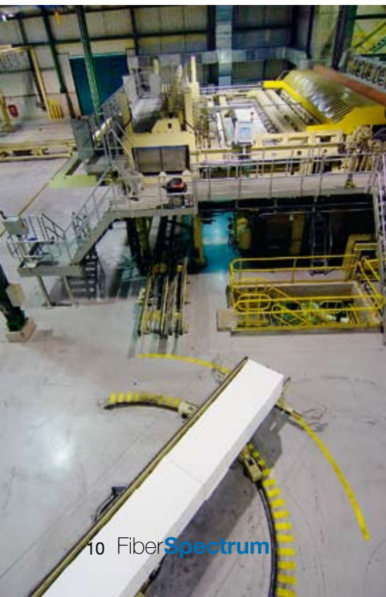
▼ The pulp drying/baling plant consists of a stock approach system with six-stage screening, a 9.23 m wide pulp drying machine, and a cutter/layboy with three automated baling lines (shown here).
