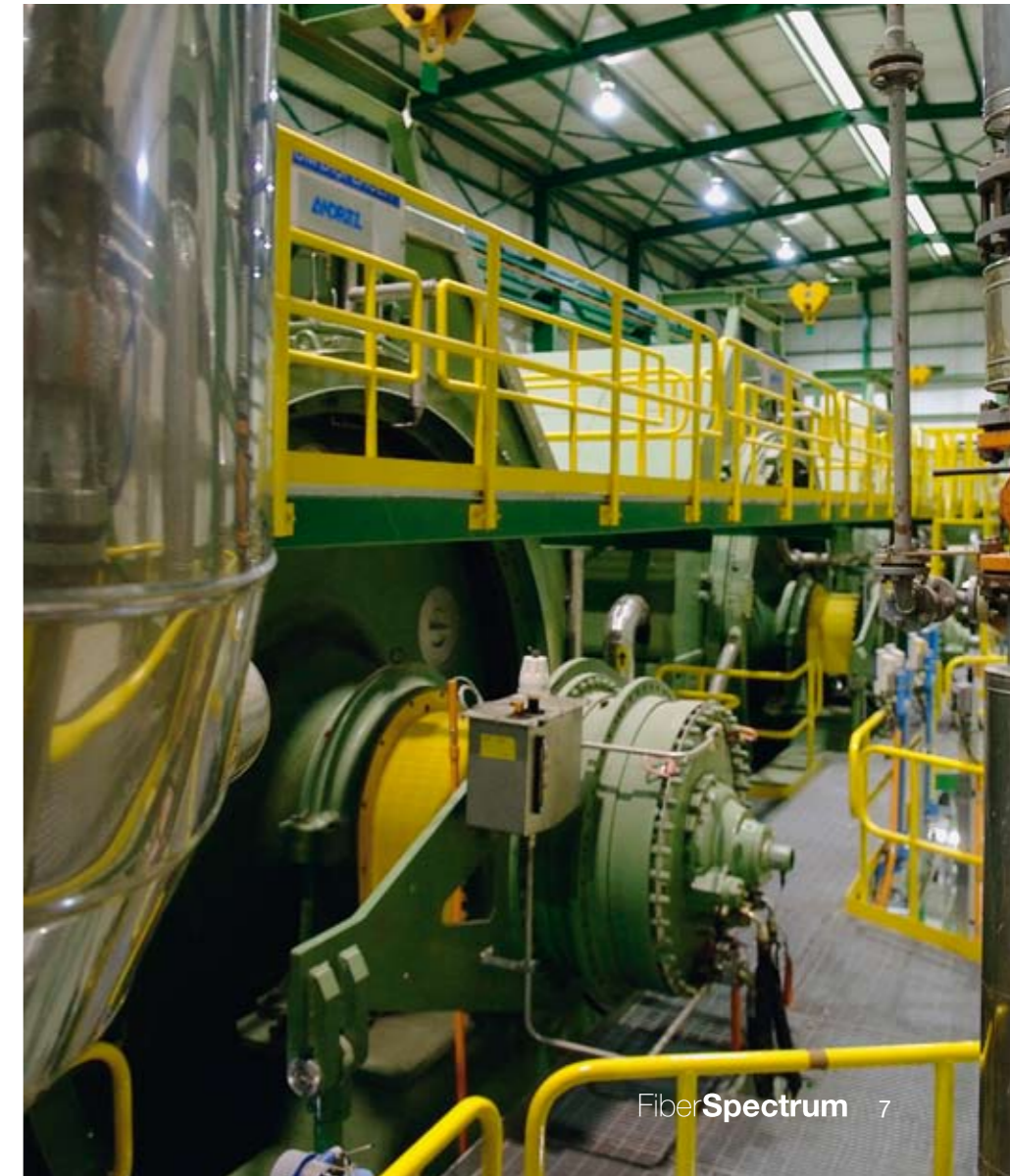
▼ The fiberline utilizes DD washers for all washing stages. A special concern during the system design was the requirement to operate the plant with 100% eucalyptus nitens pulp, which has lower drainage. After conducting mill trials on Line 1, Andritz sized the DD washers for all washing stages to be 15% larger than would be required for other eucalyptus pulps.
