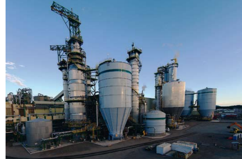
▲ The 2405 adm/d fiberline consists of a Lo-Solids® digester with TurboFeed™ chip feeding, brownstock washing, oxygen delignification, post-oxygen pulp screening and washing, and four-stage ECF bleaching.
