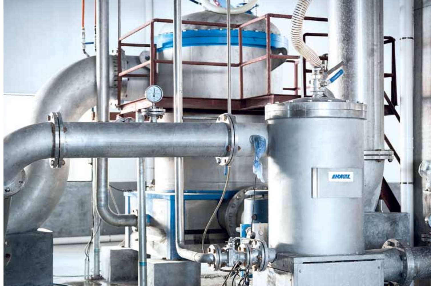
▲ A complete paper machine approach system from ANDRITZ is also in place. A ModuScreen headbox screen plays an important role in delivering stock to the new machine.
