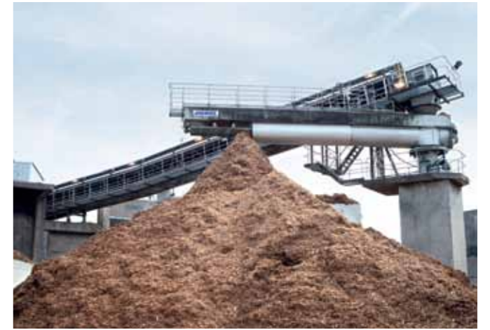
▲ The biomass is a combination of pine, spruce, and birch bark. ANDRITZ delivered a complete biomass handling and conveying system.
