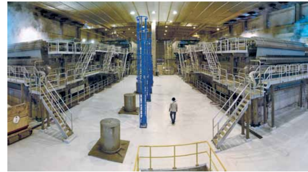
▲ ANDRITZ delivered the two-machine pulp drying plant with automated baling lines.
