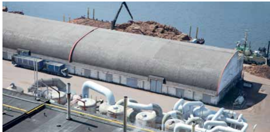
▲ A birds-eye view of the ANDRITZ evaporator line (in the foreground) that contains the Duct Stripper.
