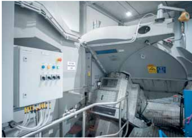
▲ There are two parallel HHQ-Chipper units at Skoghall – one for kraft and one for CTMP chips. A unique switching arrangement allows logs to be easily conveyed to either of the chippers depending on production needs.
