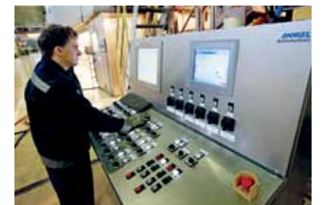
▲ ANDRITZ Automation integrated existing and new features into its DCS and QCS systems.
