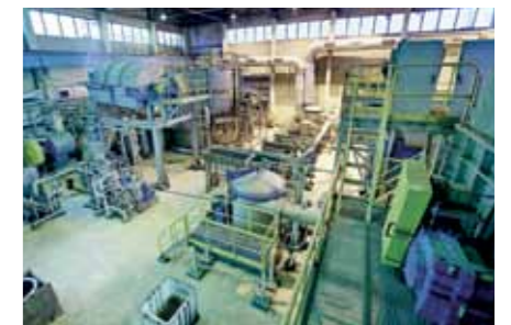
▲ ANDRITZ also delivered a new recycled fiber processing line and machine approach system with a capacity of 800 t/d to bring high-quality stock to PM7’s new headbox.
